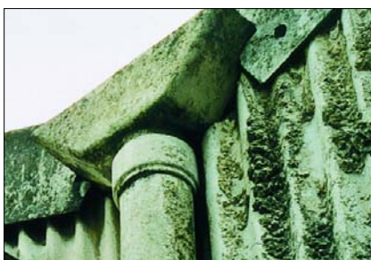
Moss and lichen growth on asbestos cement
