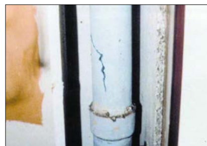
Sometimes, the joints are sealed with asbestos string.
